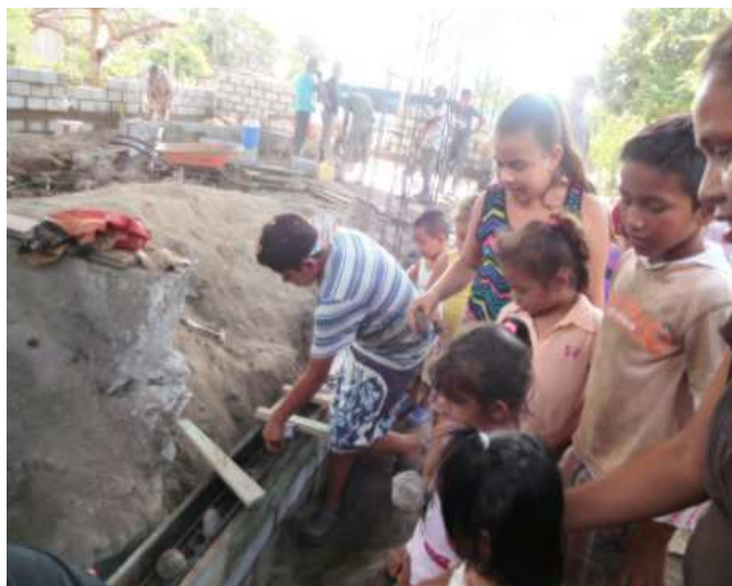
The children placing small rocks in the foundation to remind them that they are part of this church.
