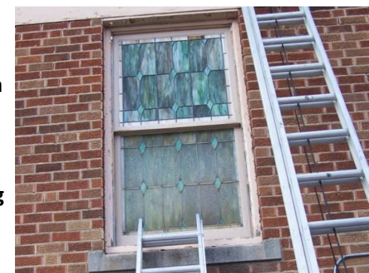
Job done ~ upper window has all new glass. The bottom window is the original at Brotherhood
