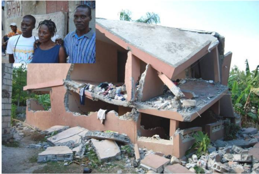
This family loses the house that missionary Bonite Affriany built for them. They are among many that will now live in tents
