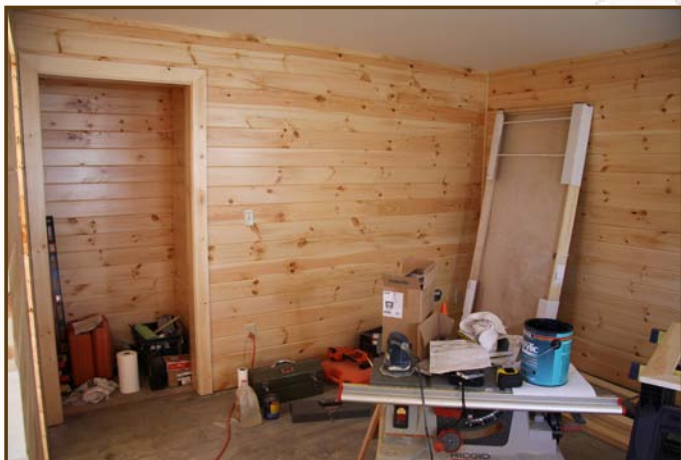
Cherokee B is in the process of a complete interior renovation with pine siding and a new bathroom.
