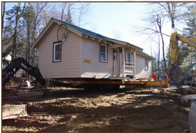
Cherokee A received major renovation work for Summer 2010 and will now be shifted slightly and brought down closer to the road, providing easier accessibility.
