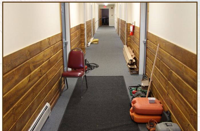
ZEITFUSS LODGE: Wood paneling is being added to the main hallway and stairwell to eliminate the need for ongoing patching & painting caused by the high use of this building.
