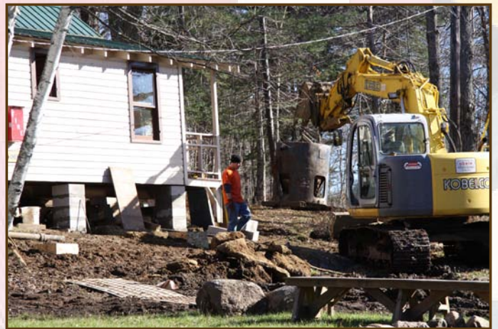
We are happy to announce that Cherokee C, a staff housing unit in 2010, will be fully renovated and available as a two-bedroom accommodation for guests in 2011.
