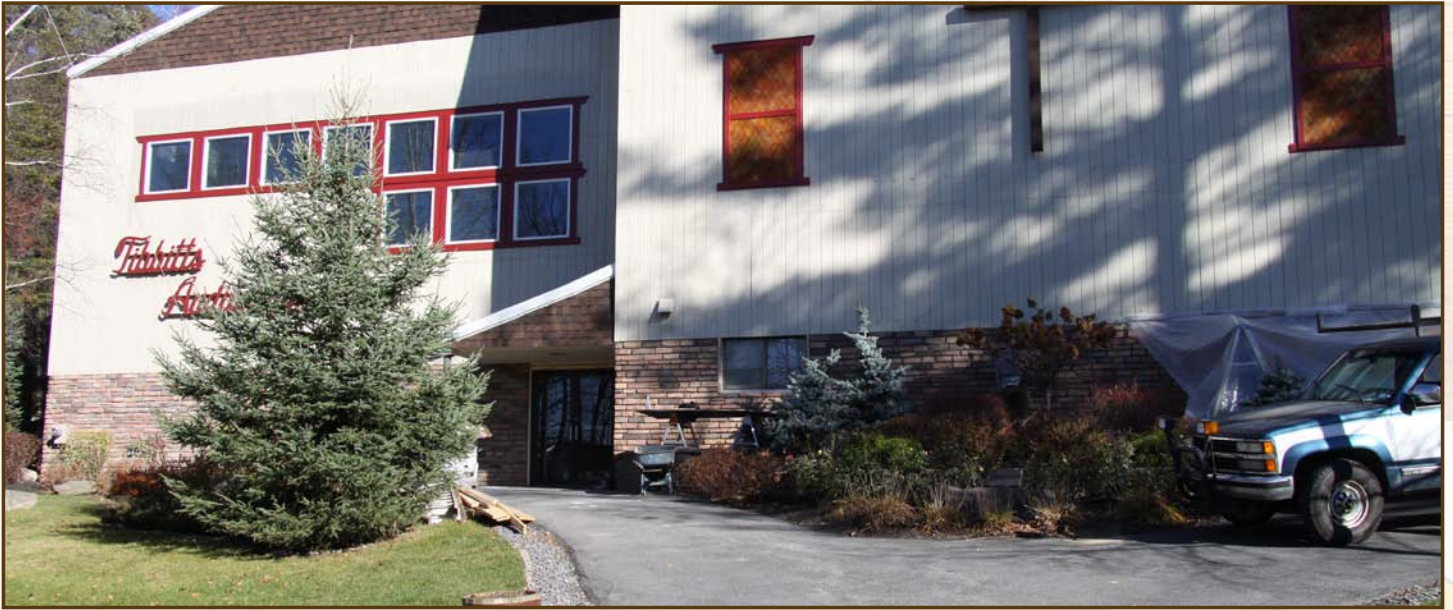
TIBBITTS EXTERIOR: Our key worship facility, located in the center of Camp, is receiving a new stone facade around the front exterior, as well as new vinyl siding.
